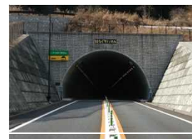
Number of Road Tunnels 562 (as of Mar 31, 2021)
